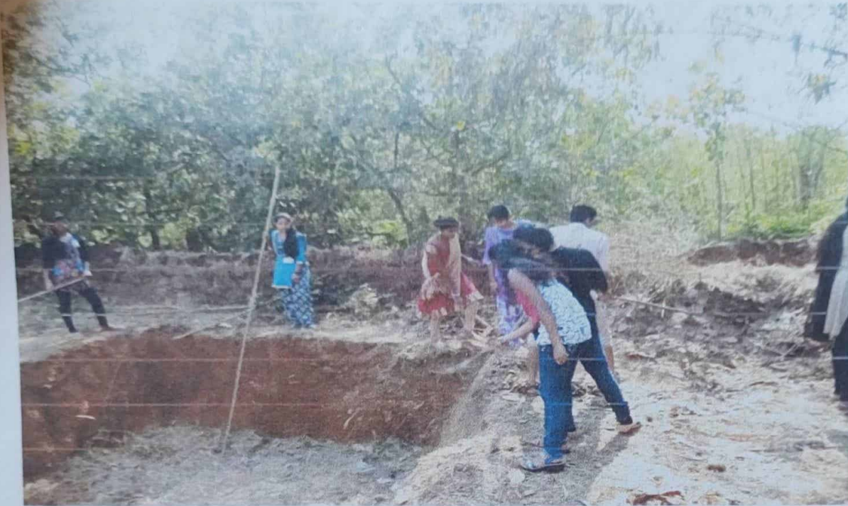
Soak Pit in College
